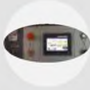
PLC Kontrol Panel PLC Control Panel
