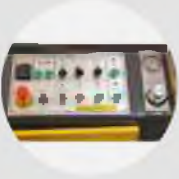
Kontrol Panel Control Panel
